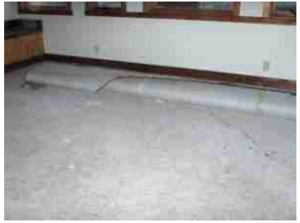
(1756 Sapphire Ranch Trail water damage in master bedroom.) i262854CE
