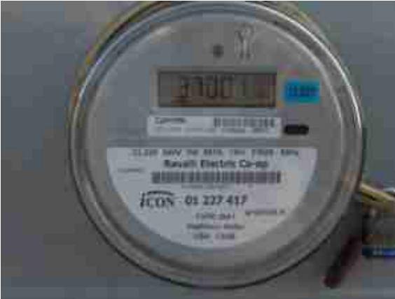
(1756 Sapphire Ranch Trail Electrical Meter)
