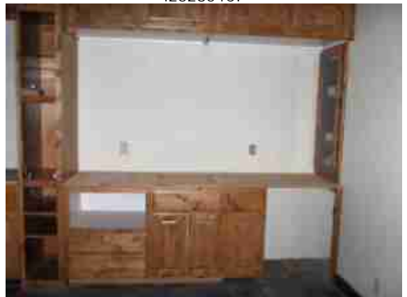
(1756 Sapphire Ranch Trail missing counter top and outlet cover.)
