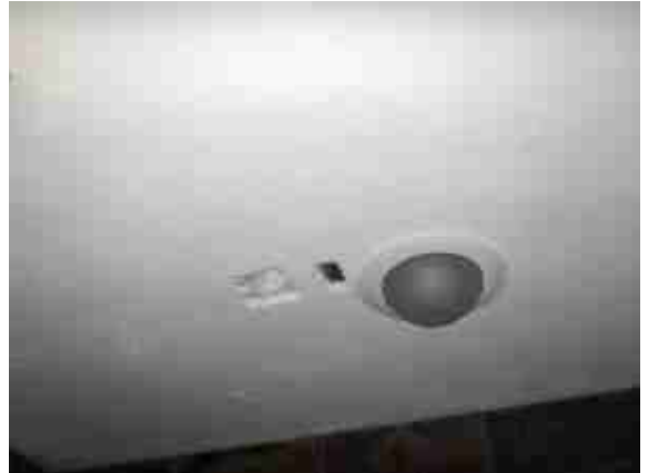
(1756 Sapphire Ranch Trail hole in bedroom 2 bathroom ceiling.) i262854CG
