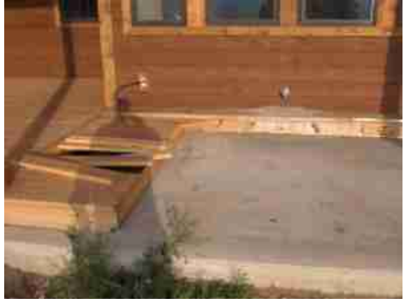
(1756 Sapphire Ranch Trail missing portion of deck)
