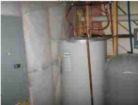
(1756 Sapphire Ranch Trail hot water tank.) i262854CH
