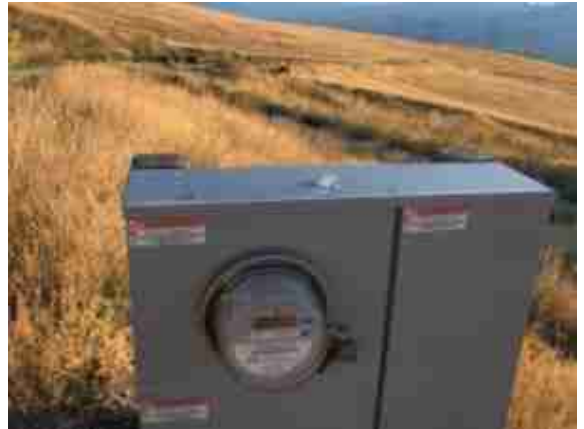
(1756 Sapphire Ranch Trail key taped on electrical meter box.) i262854BY
