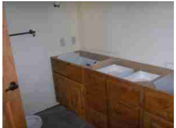
(1756 Sapphire Ranch Trail theater room bathroom with missing counter top and sinks.) i262854BU
