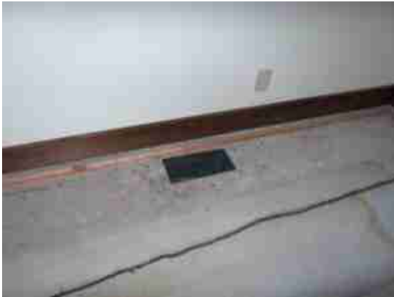
(1756 Sapphire Ranch Trail vent cover open and more evidence of water damage.) i262854CF
