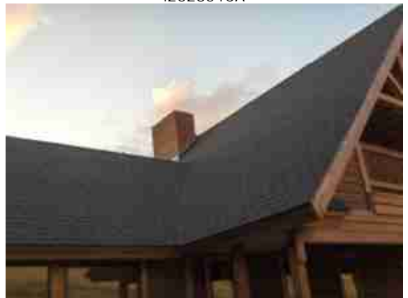
(1756 Sapphire Ranch Trail missing chimney cover.) i262854CC
