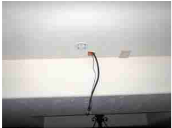
(1756 Sapphire Ranch Trail loose wire hanging from ceiling in game room.)
