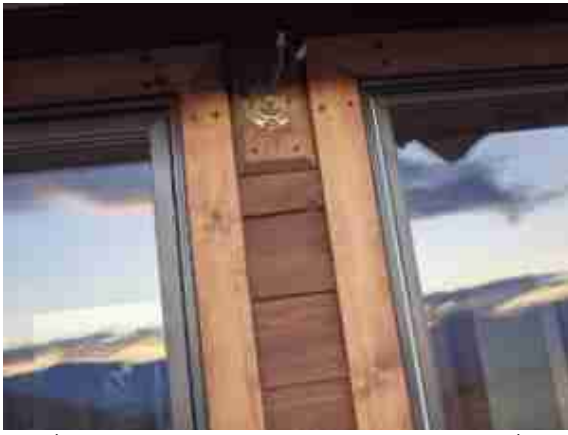
(1756 Sapphire Ranch Trail missing fixture.) i262854CD
