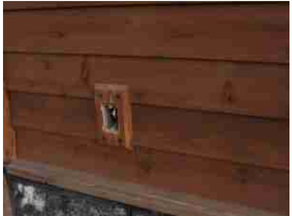
(1756 Sapphire Ranch Trail missing fixture/outlet.)
