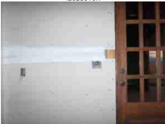
(1756 Sapphire Ranch Trail missing covers/fixtures in garage.)
