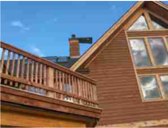
(1756 Sapphire Ranch Trail chimney cover blown loose.)
