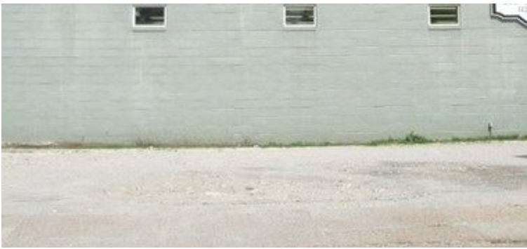
gravel parking lot showing deferred maintenance
