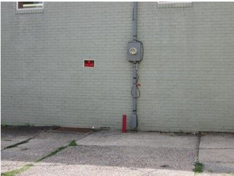
cracked cement area next to right side of building (posted no parking)
