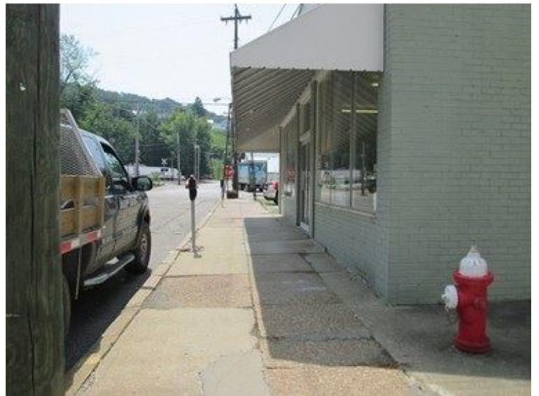
sidewalk in front - trip/fall hazard (owner husband claimed maintained by town)
