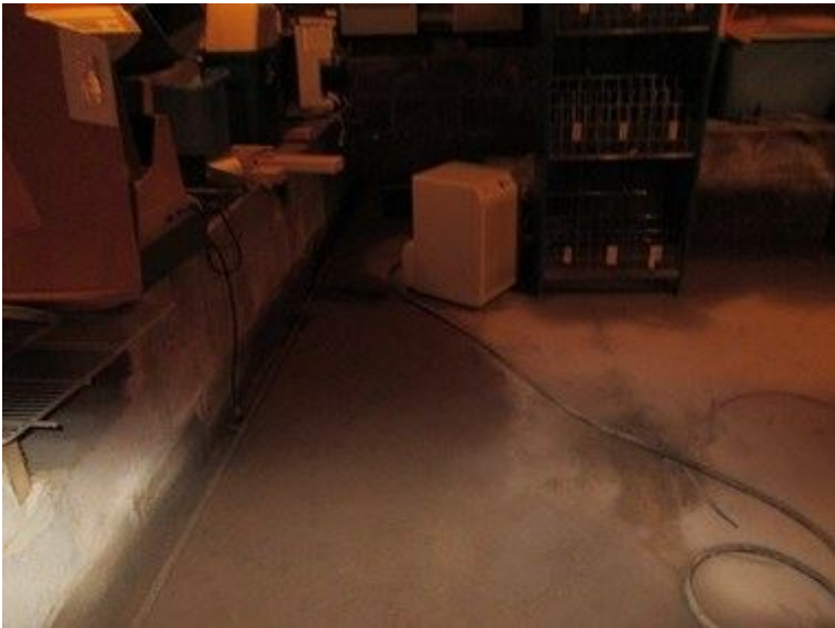
basement: water seepage from rain (damp afterward)
