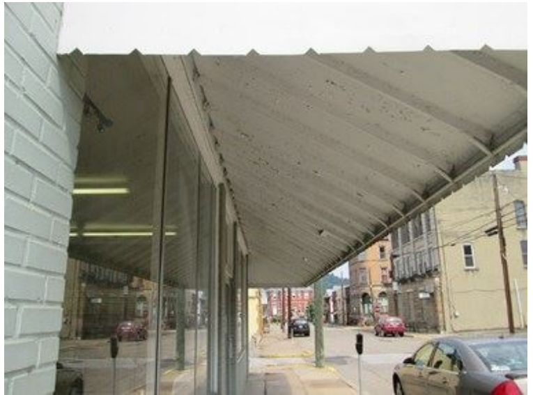
awning (peeling paint hazard)
